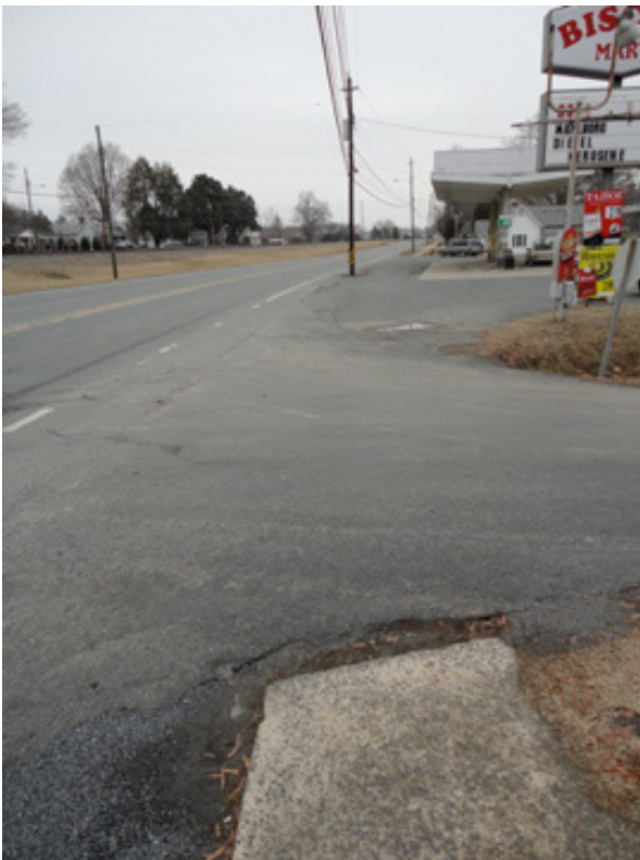
Sidewalk is found on both sides of this roadway crossing and Biscoe Mart convenient store driveway. In-between is a lack of safe, separated pedestrian space. The location above is South Main Street at Hyde Street.
