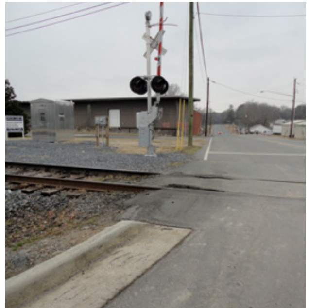
Sidewalk along Mill Street stops at the top of this picture before reaching the railroad crossing, near South Main Street. This railroad crossing is not adequate for pedestrians.
